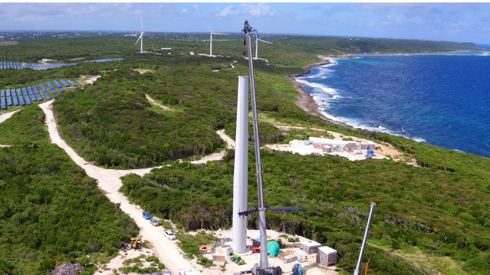
Installation work with the main crane on a LEITWIND wind turbine of the type LTW80 1.65MW Typhoon
